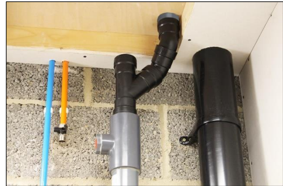
23. The combination of the T-piece and the two 45° connectors allow manipulation of the constructed coupling to achieve multiple positions to connect to the shower waste pipe.
